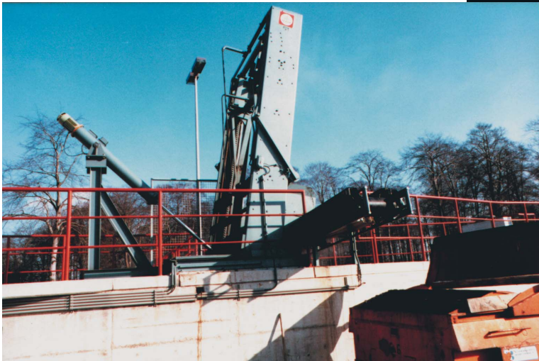
Clarification plant Actuator for rake control
