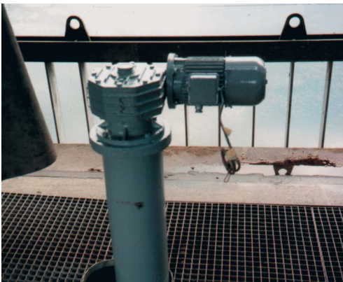
Flood gate actuator
