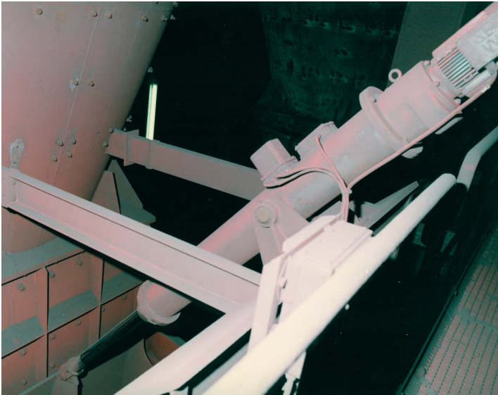
Bunker flap control in steel plant
