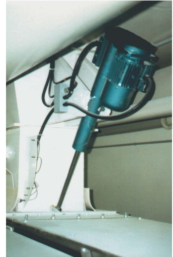
Silo feeding installation for belt conveyor system
