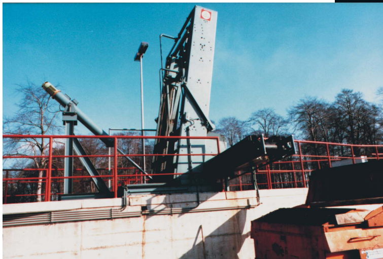
Clarification plant Actuator for rake control
