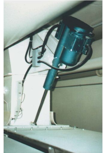
Silo feeding installation for belt conveyor system
