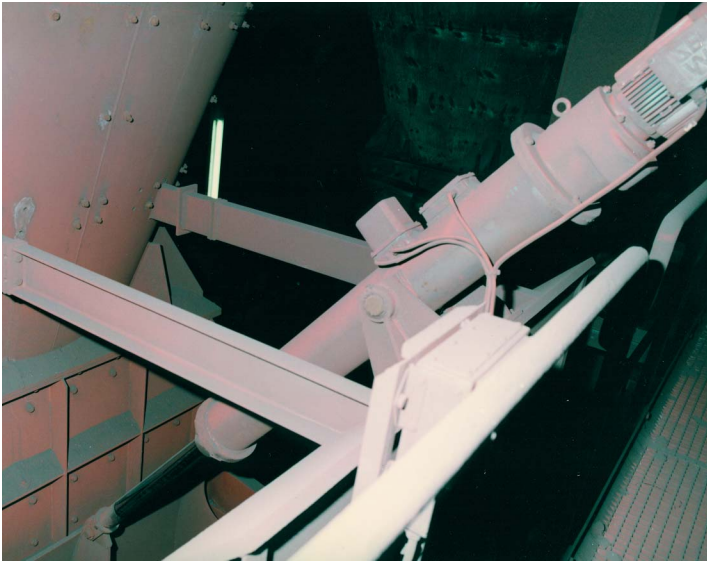
Bunker flap control in steel plant
